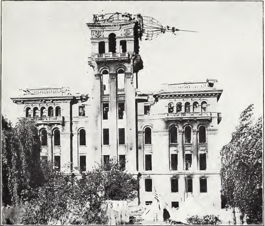
A. WRECKED TOWER AND SPALLED STONWORK, HALL OF JUSTICE, SAN FRANCISCO. Photograph by John Stephen Sewell.
